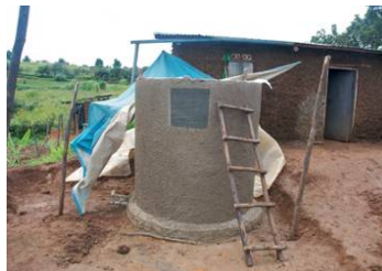
Figure 45 : Cuve en ciment (ferrocement tank) (source : Kigezi Diocese WSP)
